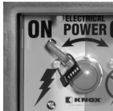
Lock-out/Tag-out posts accommodate a tamper seal
