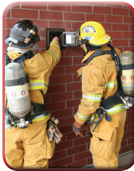
Firefighters Blocker and Emmons accessing the Knox-Vault at the new high school.
